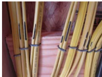
Cables marked with black marker
